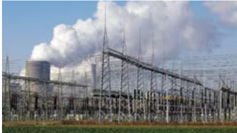
▲ The electricity you use probably comes from an electrical power plant like this one.
